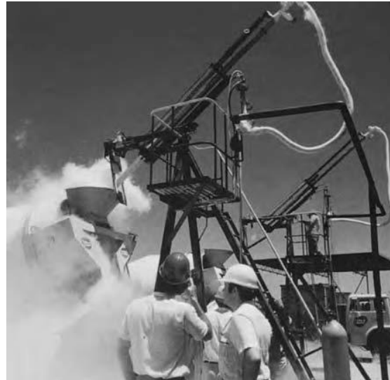
Figure 18.4 – Injection of Liquid Nitrogen into an Agitator Truck to lower Concrete Temperature
